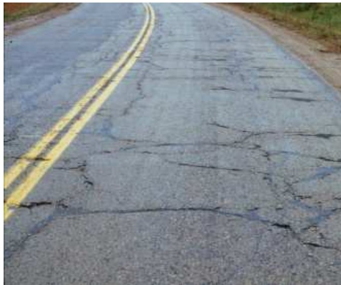
Figure 2.9 Cracking permanent deformation. [6]
