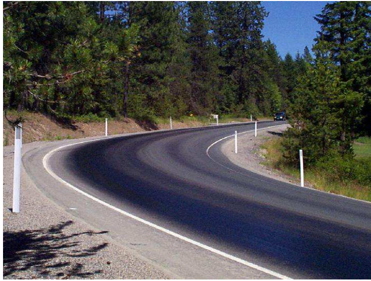
Figure 2.10 Bleeding permanent deformation. [6]
