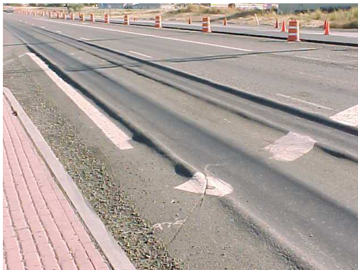
Figure 2.8 Rutting permanent deformation. [6]
