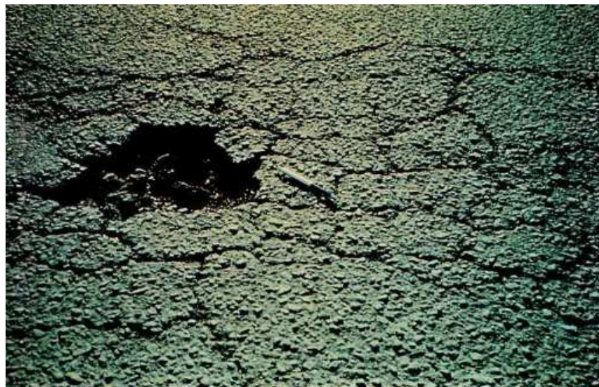
Figure 2.11 Potholes permanent deformation. [6]
