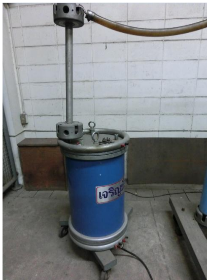
(a) HV test transformer
