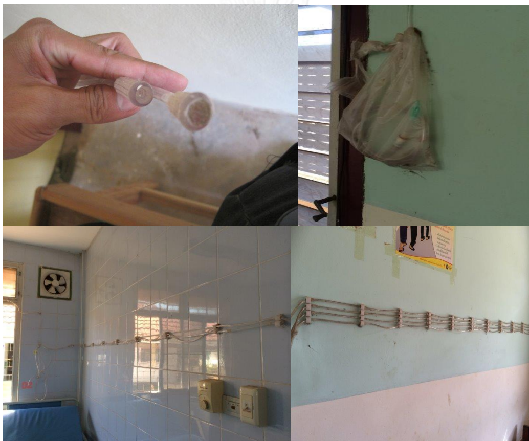
Figure 12: Oxygen tubing and tubing outlet
