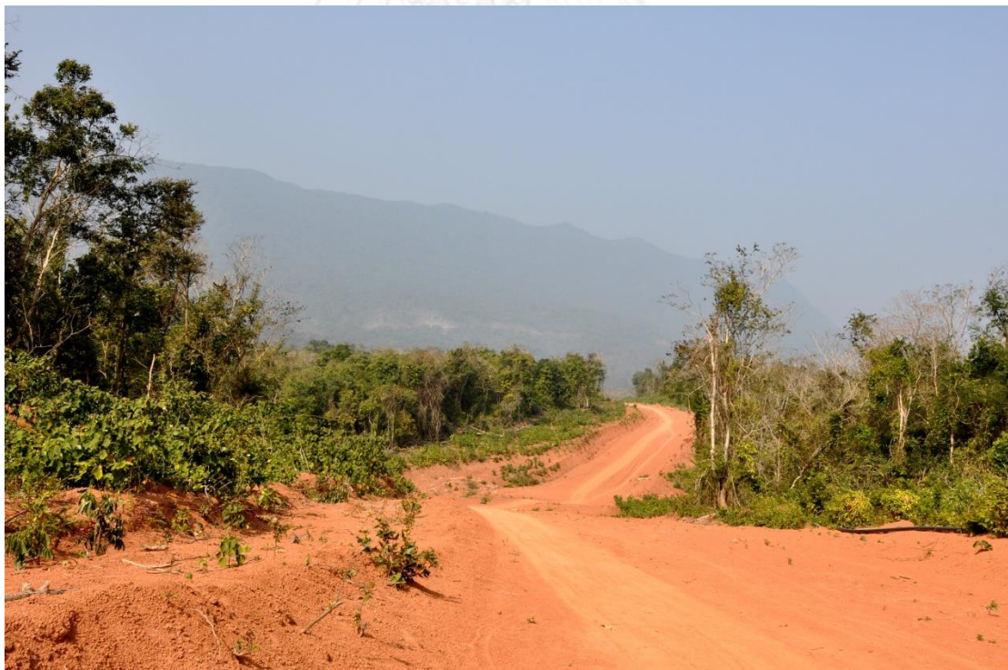
A new road being cut to Mu Gia Pass in early 2014. Existing Route 12 can be seen in the background. It is the white cut into the green mountainside above the new road Photo by Mick Elmore
