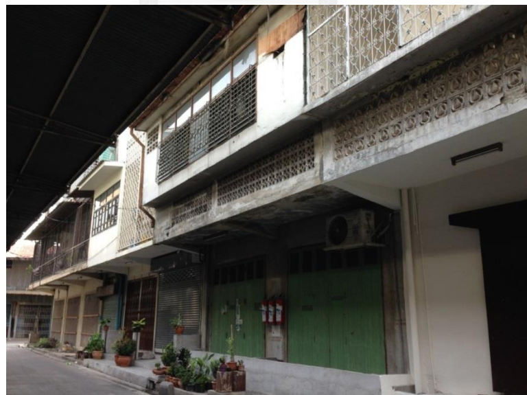
Figure 3. 47 Corridor has been sealed with solid wall and windows can provides more space and security.
