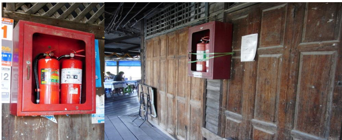
Figure 3.4: Fire Extinguisher on the wall of most coner in Bang Pli Water Market. Photo taken by the author
