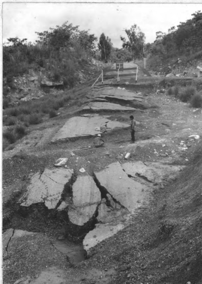
Figure 2.6 Failure of the embankment in August, 1986.
