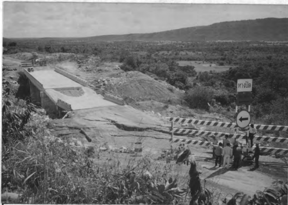
Figure 2.2 Second failure on the bridge and bridge approached abutment between KM. 12.696 and KM. 12.745.
