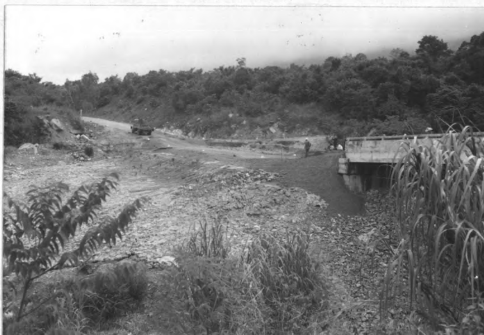
Figure 2.5 Initial failure of embankment in August, 1985.
