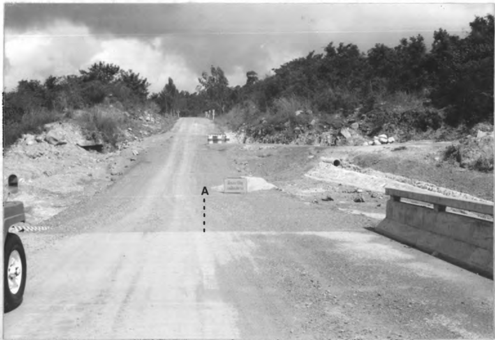
Figure 2.4 Remedial measure of second failure in 1983.
