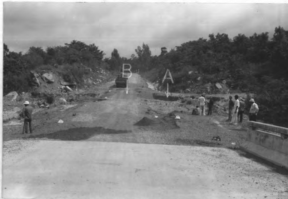
Figure 2.8 Major crack of failure in 1985.
