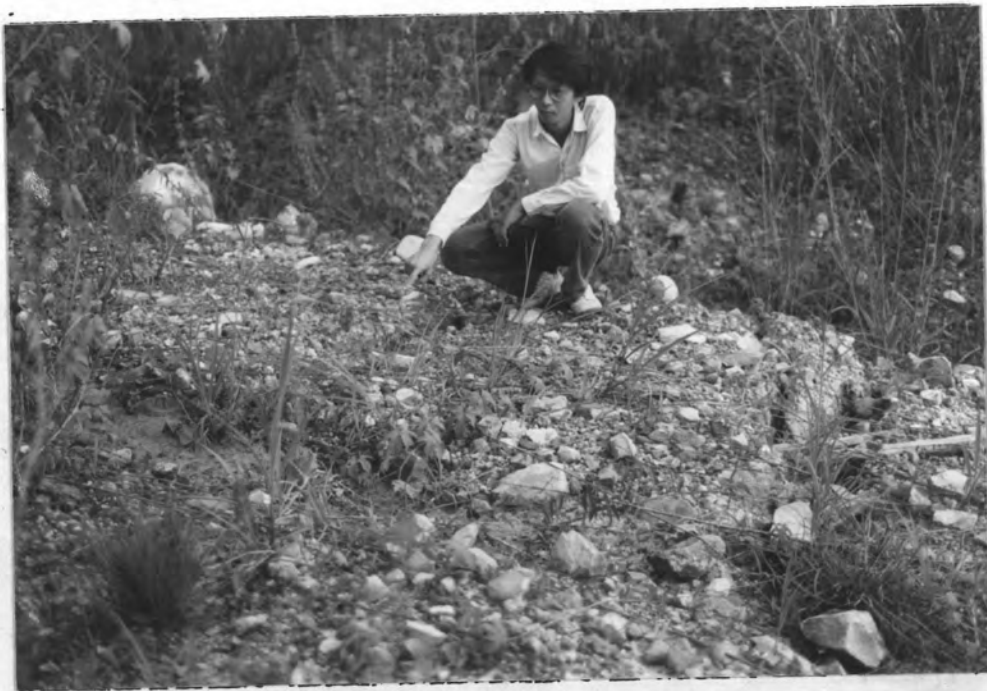
Figure 2.10 Tension cracks in the colluvial slope near the toe of the embankment slope
