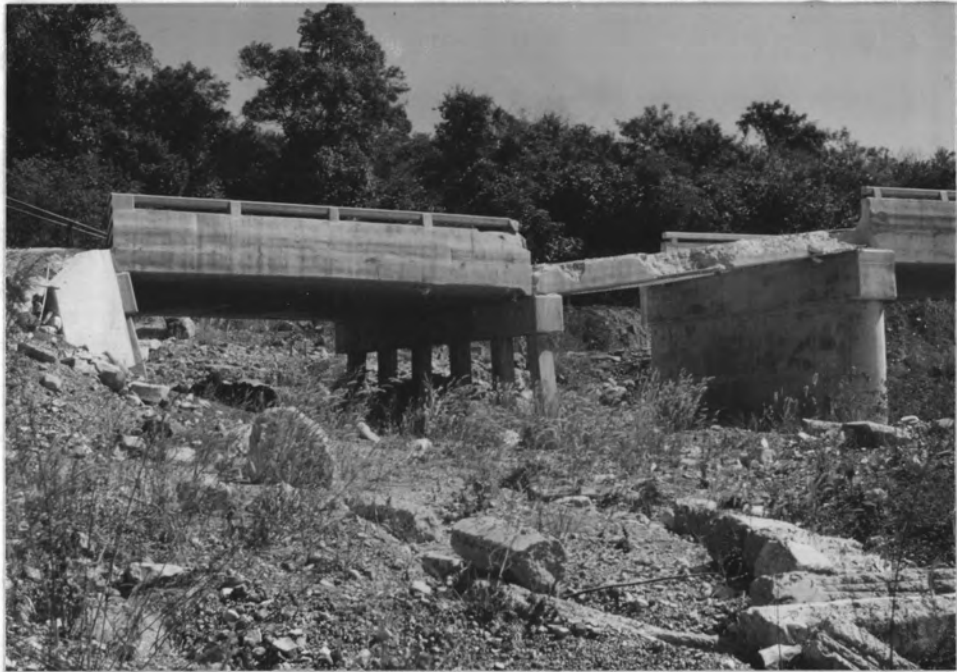
Figure 2.2(cont.) c) Damaged bridge between KM. 12.696 and KM. 12.714
