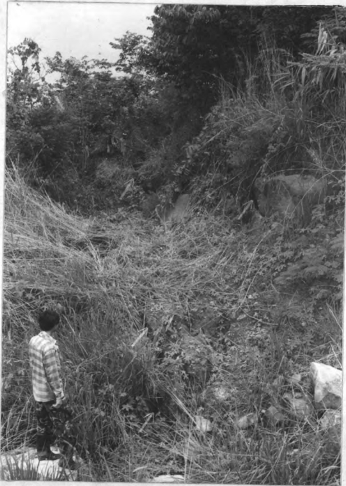
Figure 2.12 Fresh soil movement (at the arrow point) at the natural landslide scarp.
