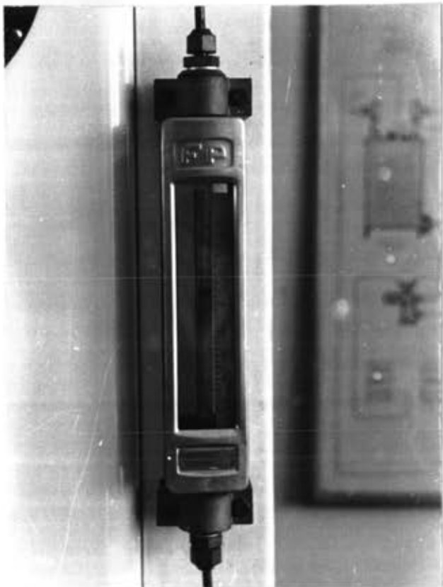
PHOTOGRAPH 4 Refri- gerant liquid flow- meter.
