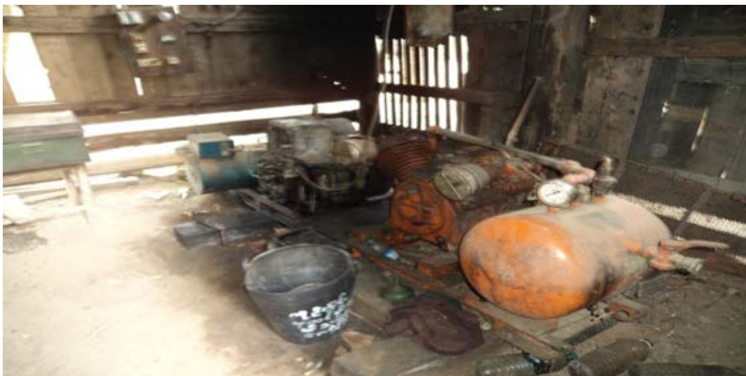
Picture 5.3: Diesel generator in Mone Taw monastery (author's photograph)
