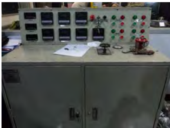
Figure B-3 A dynamometer's controller
