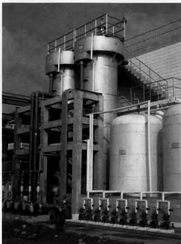
Figure 2.3 Fluidized-bed Fenton reactor in full-scale.
