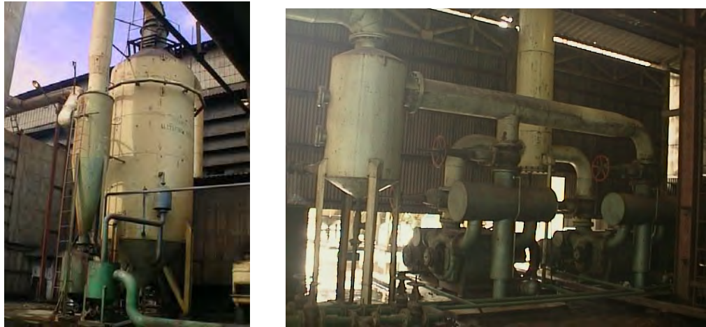
Figure 2-8 :CO2 gas purification and compressor
