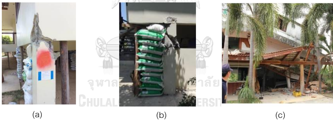
Figure 1.4 Building damage (Ruangrassamee et al., 2014)
