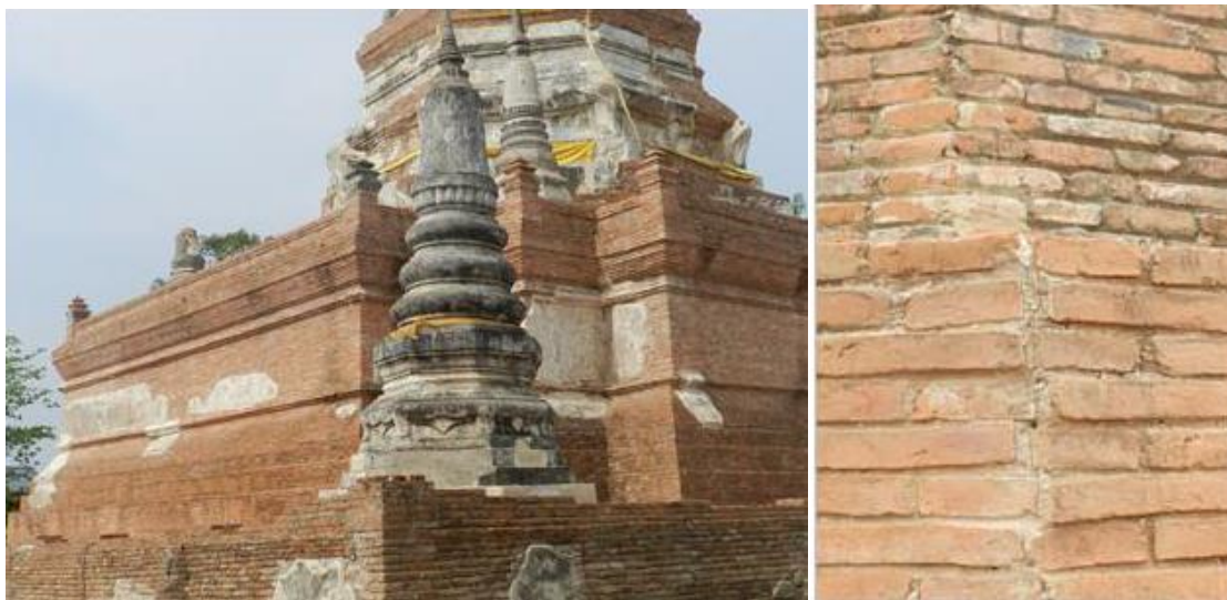
Figure 25 ICOMOS experts point out extensive reconstruction and poor masonry skills Source: Nishiura and Dilawari (2014)
