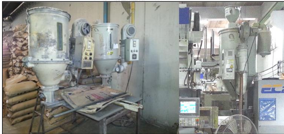
Figure 3-2: Ground hopper drier and overhead hopper
