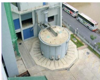
Storm Pumping Station
