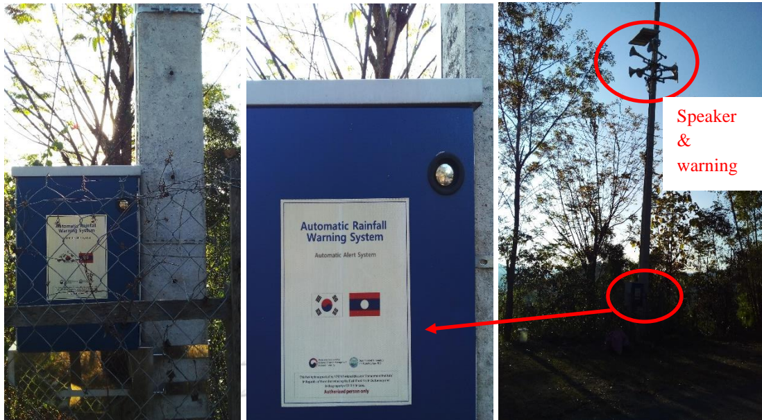
Figure 4.11: The early warning system sensor and equipment at Thin village.
