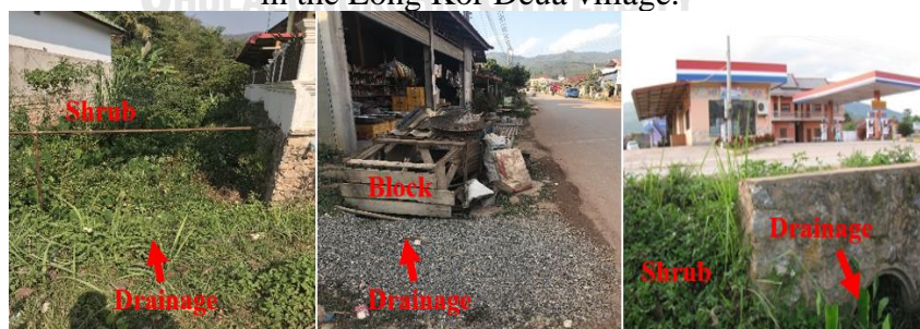
Figure 4.14: the drainage status in the Long Kor Deua village.
