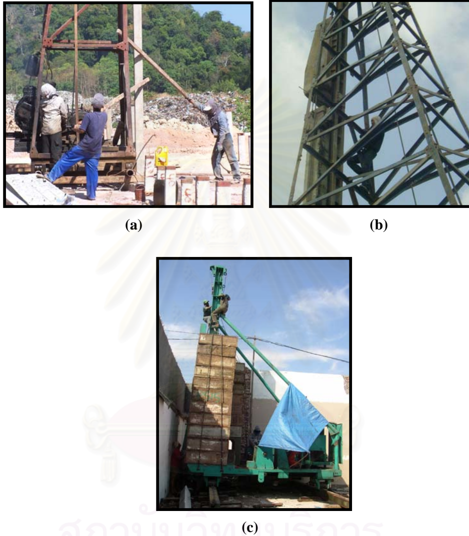
Figure 5.15 Improper work method of Malaysian drop-hammer (a), Thai drop-hammer (b) and Indonesian pile-pushing machine (c).
