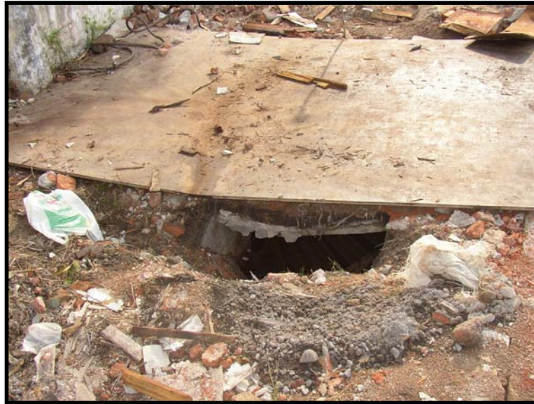
Figure 4.20 A bended support base of a pile-pushing machine after used near a hole
