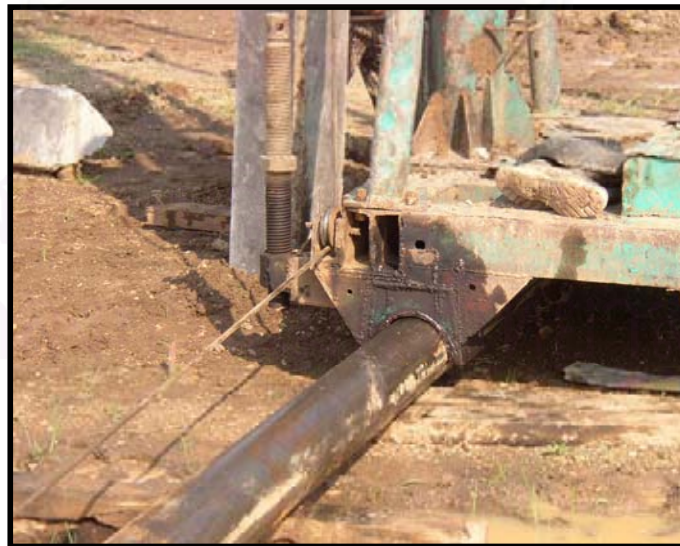
Figure 4.11 Mechanism of shifting an support using an attached hoist at Indonesian drop-hammer
