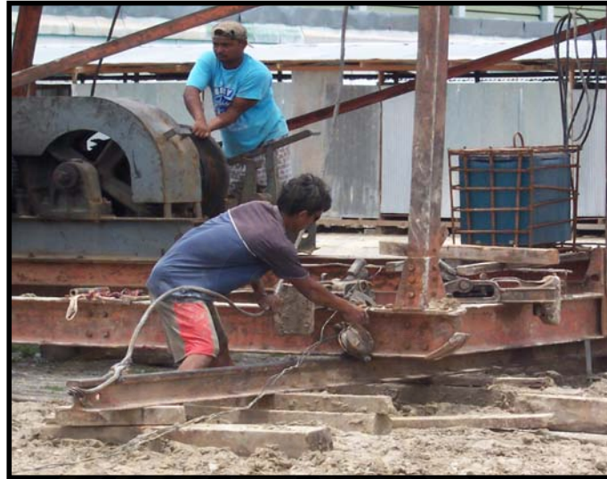
Figure 4.12 Mechanism of shifting an support using a moveable hoist at Thai drop-hammer
