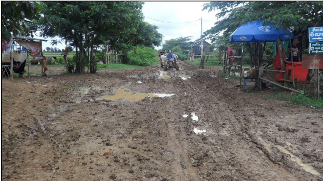
Photograph 1: An image of road condition in Prek Trob village after raining
