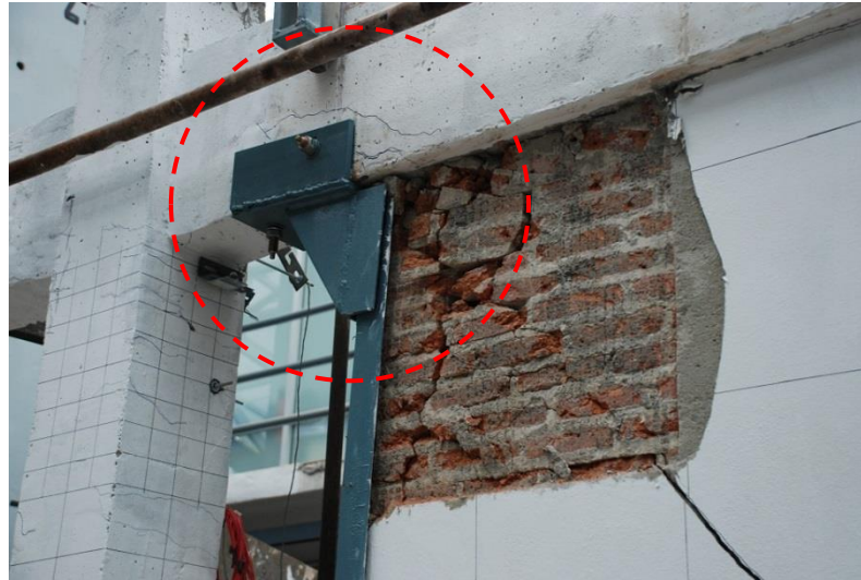
Figure 4-11. Damage condition in the RC beam of specimen MIRCF02 at 2.00% drift
