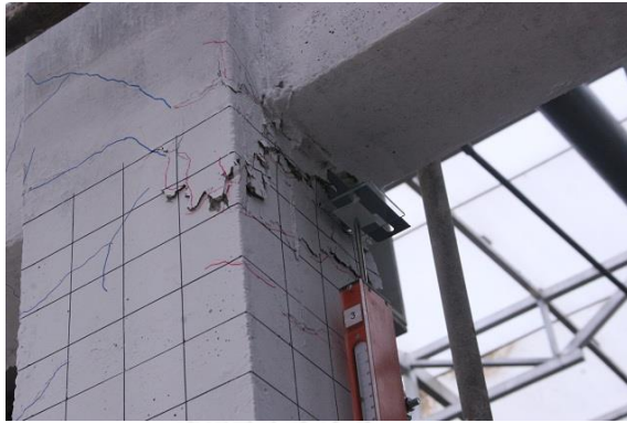
Figure 4-15. Splitting of concrete in the RC column at 1.75% drift
