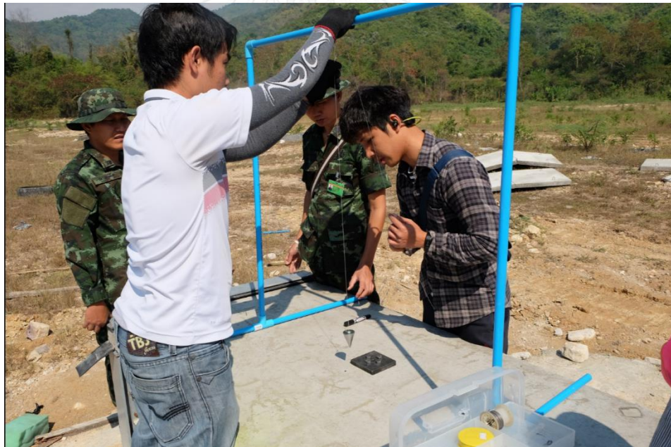
Figure 3.1-8 Use of pendulum to ensure that the explosive is right above the center of the panel
