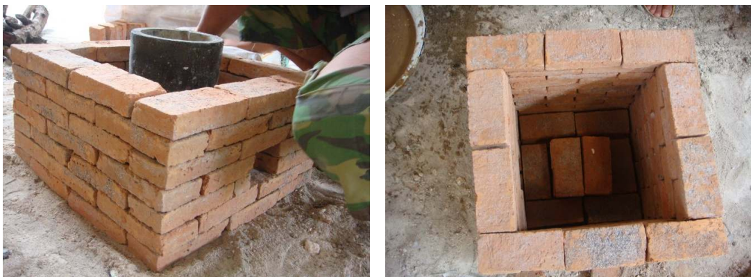
Figure186 Making brick furnace with air hole at the bottom to melt bronze.
