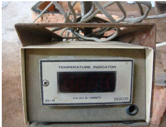
Figure178 Monitor of temperature indicator.
