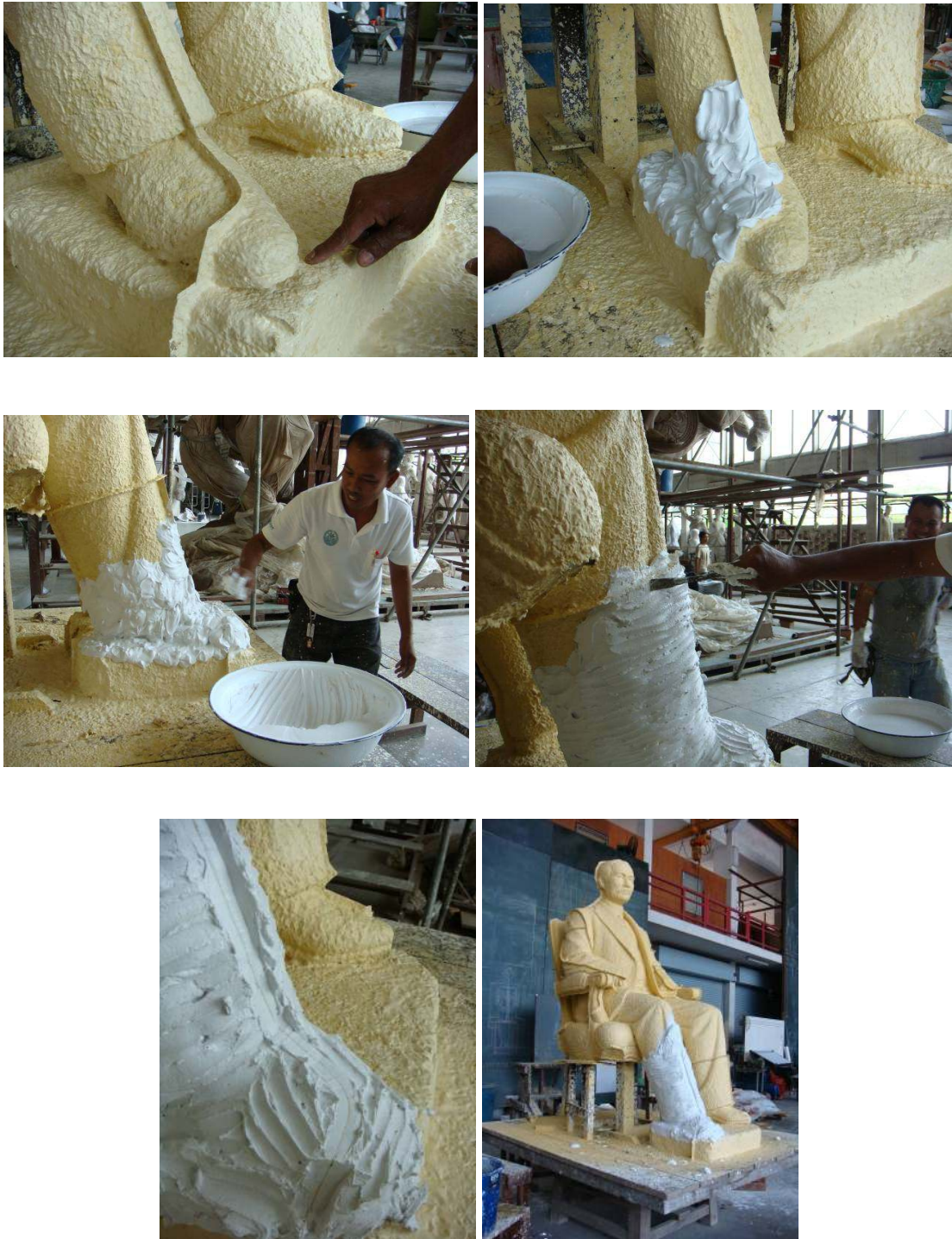
Figure 39 Applying Gypsum plaster paste on the statue and revealing the edge of zinc plates
