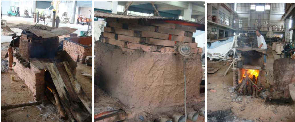
Figure183 Increase fire heat until the fire ball stops to appear from the mould.
