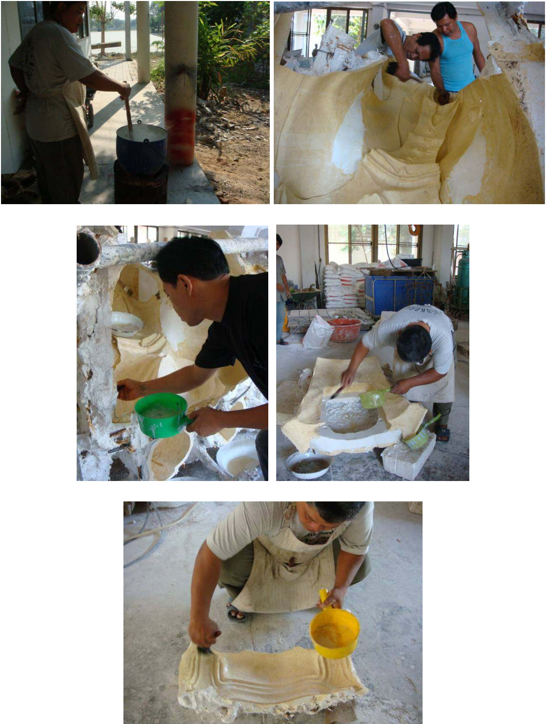
Figure 54 Boiling coconut oil and Soap solution to apply on the plaster mould.
