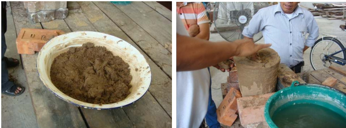
Figure168 Fill the hole on the base with clay and sand mixed plaster.
