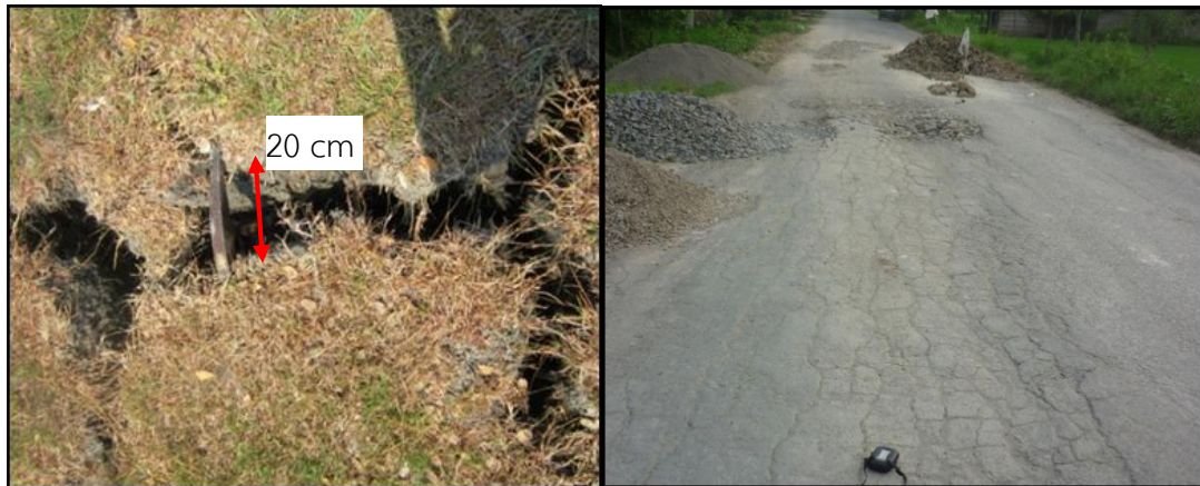
Figure 2-6: Deformation and cracking of road structure during dry season, Ngawi, Indonesia (Por & Karnawati, 2012).
