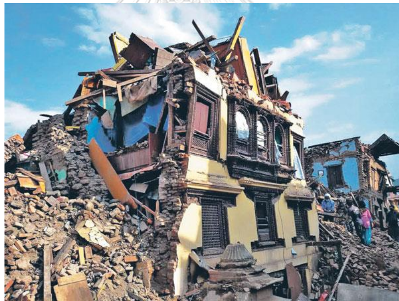
Figure 5: Houses destroyed by the quakes in Sankhu Source: (Una, 2015)
