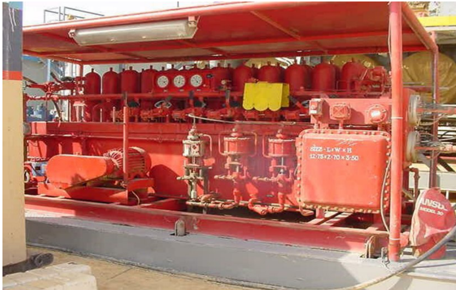
Fig 100: Accumulators and BOP control system
