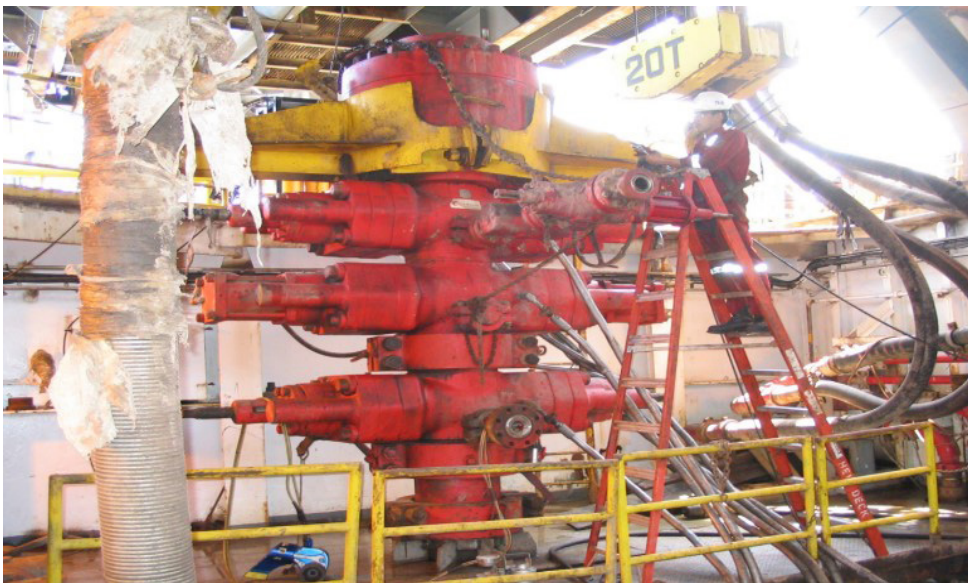
Fig 91: Blowout preventer stack
