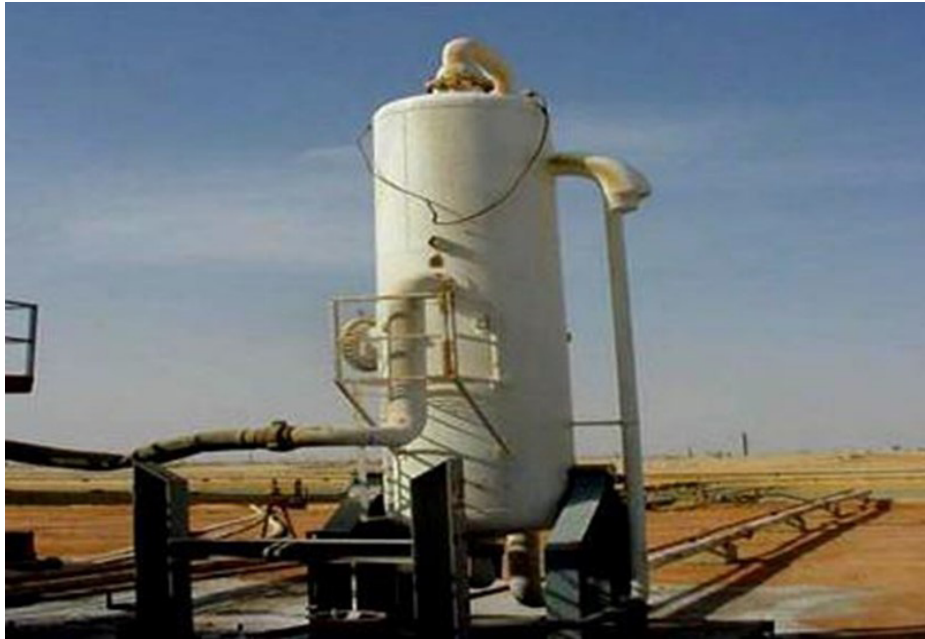
Fig 102: Mud gas separator
