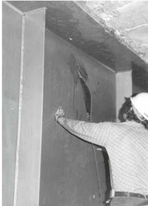
Figure 1.1 Full girder depth fatigue crack of Lafayette Street Bridge in St. Paul, MN (Dexter and Ocel, 2013).
