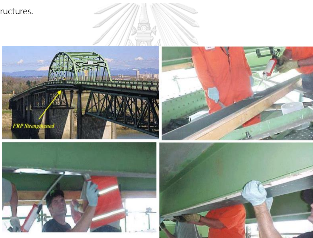
Figure 1.3 Repairing cracked steel structures with FRP patches - The Sauvie Island bridge, Portland, Oregon, USA; Mosallam et al. (2013)
