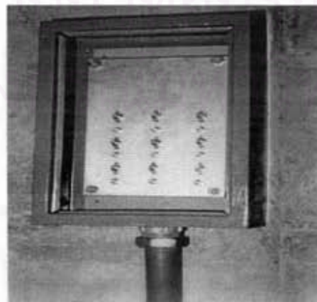
Fig. 3.3.15 Termination box, provided 9 BNC jacks
